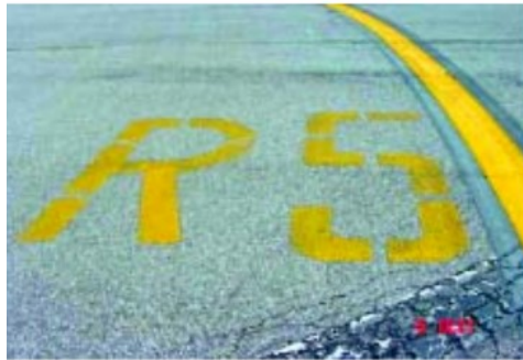
Photograph 6 Marking showing direction TWY R5.
