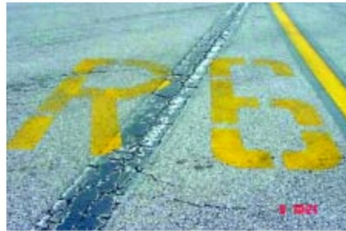
Photograph 7 Marking showing direction TWY R5.
